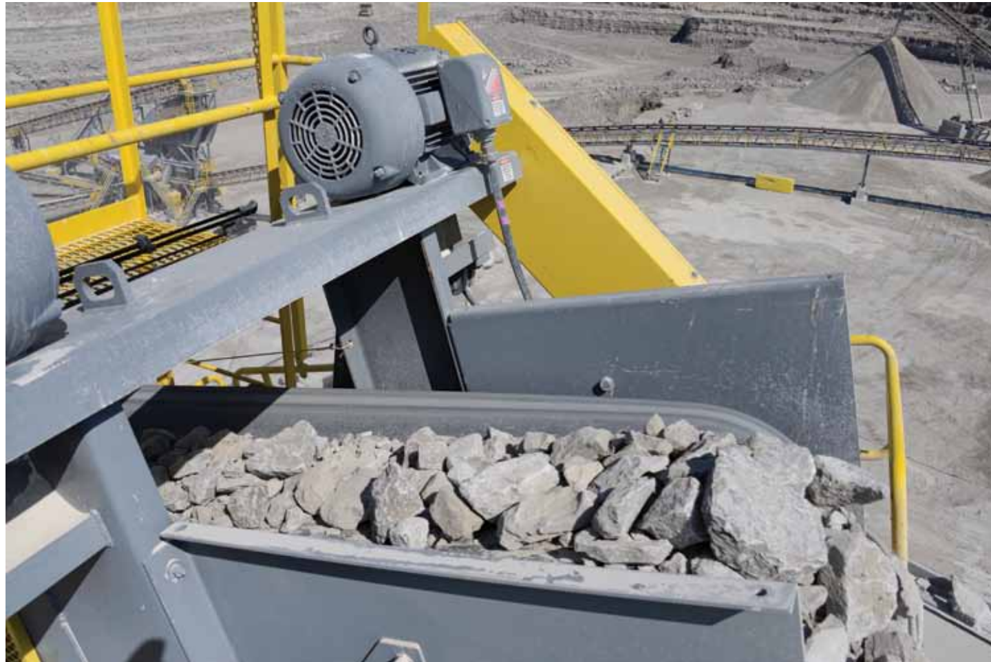
Baldor•Reliance Quarry Duty and Severe Duty motors are used throughout the Bluegrass facility. With heavy-gauge steel and cast-iron construction, these motors are designed to deliver reliable, rugged performance. Quarry Duty motors are Design C with increased starting torque, ideal for starting loaded conveyors.
